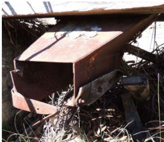
FIGURE 7.14: Close-up view of the chute from below. Photo by Brian Fox, 2015.
